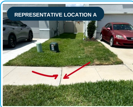
Observed sidewalk settlement at residential side-yard utility corridor.
